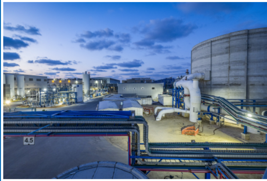
General view of a water desalination facility near Rishon LeZion, central Israel, September 2, 2026. Photo by Yossi Aloni/Flash90
